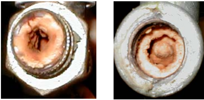
Fig. 8 the outlet pipes from the boiler for hot water
